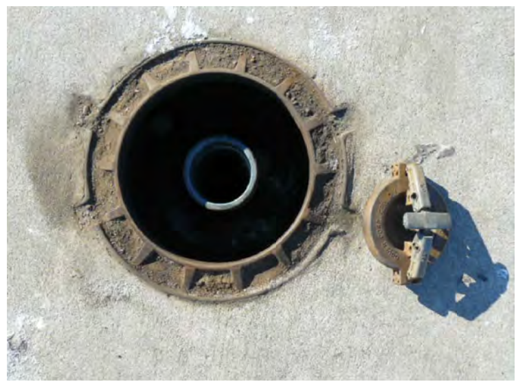
16" DIESEL AND GAS FUEL FILL MANHOLE (D & G)
