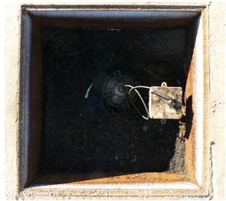
24" DIESEL AND GAS MONITORING MANHOLE (DM & GM)
