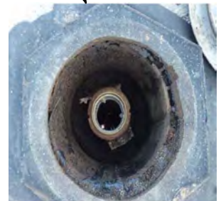
16" DIESEL AND GAS FUEL FILL MANHOLE
